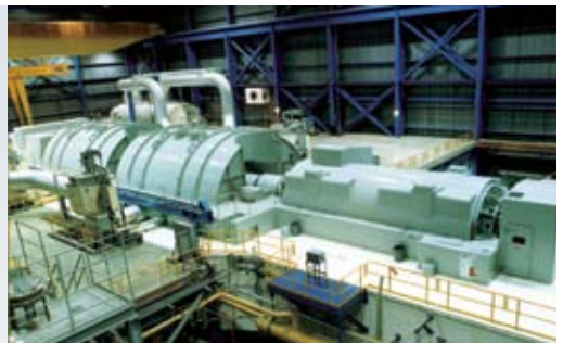
Generating unit and moisture separator-reheaters
