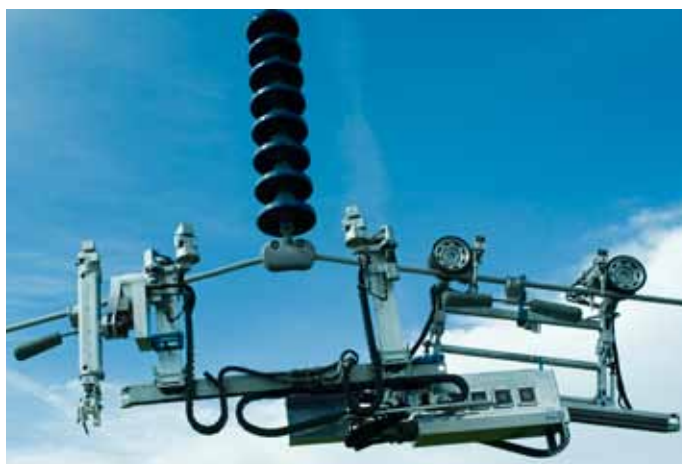
LineScout crossing an insulator string
