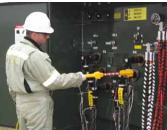
Using the Hydro-Québec sniffer on grid equipment
