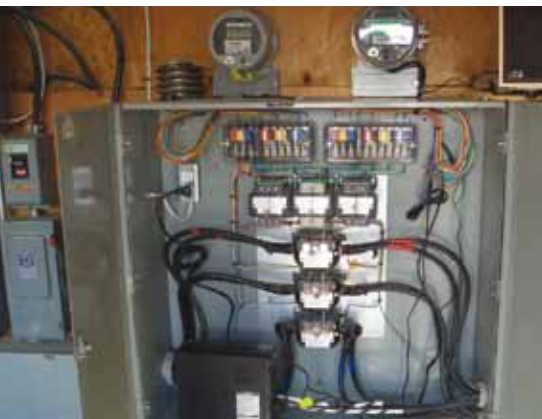
Measurement module cabinet
