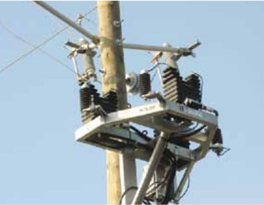
Remotely monitored voltage transformers
