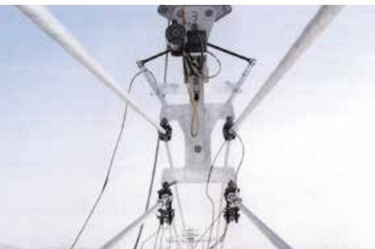
Relative displacement transducers on a quad bundle.
