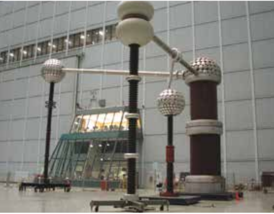
Test hall measuring 82 m by 67 m and 50 m high, insulated against radio interference (attenuation of 50 to 60 dB at 1 MHz and acoustic suppression).
