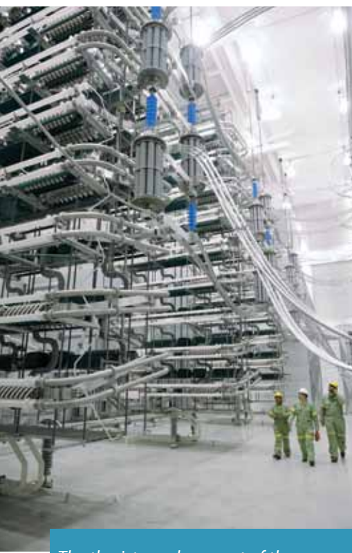
The thyristor valves, part of the converter, are the key component in the conversion operation that separates the Québec and Ontario power grids.
