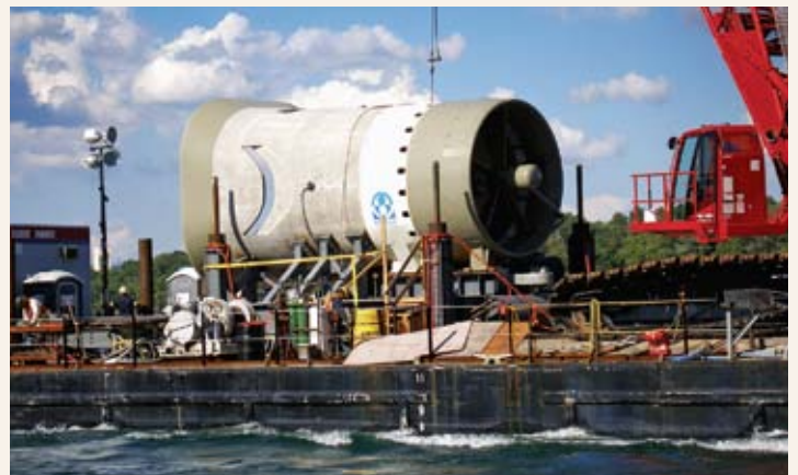
Prototype of a hydrokinetic turbine being installed in the Saint-Laurent, close to Montréal. Hydro-Québec, in conjunction with Groupe RSW, will assess the turbine's efficiency and performance.
