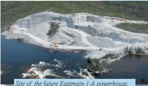
Site of the future Eastmain-1-A powerhouse, right next to the Eastmain-1 facility
