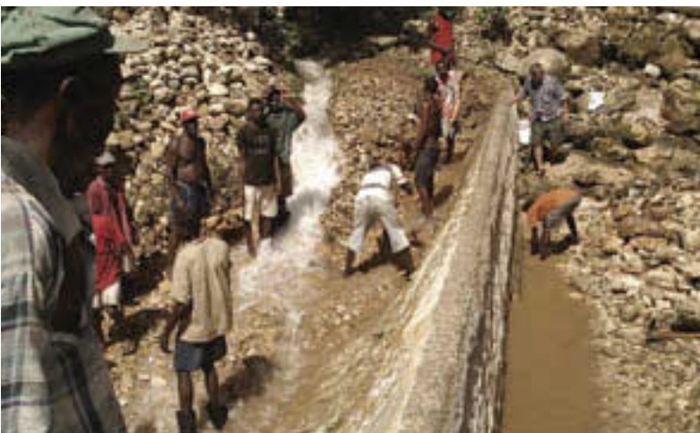
Rehabilitation of a weir at Gaillard generating station: a cooperation project in Haiti.
