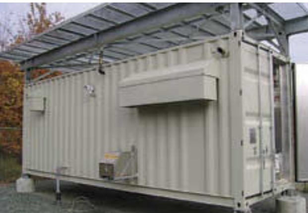
New fuel-leak detection system.
