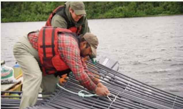
Installation of a fish barrier on the Romaine. The goal: to estimate the abundance of the adult salmon population migrating upstream in order to evaluate the impact of the operation of future generating stations.
