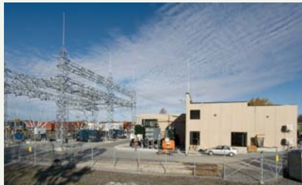
Gatineau substation, returned to service in 2009.
